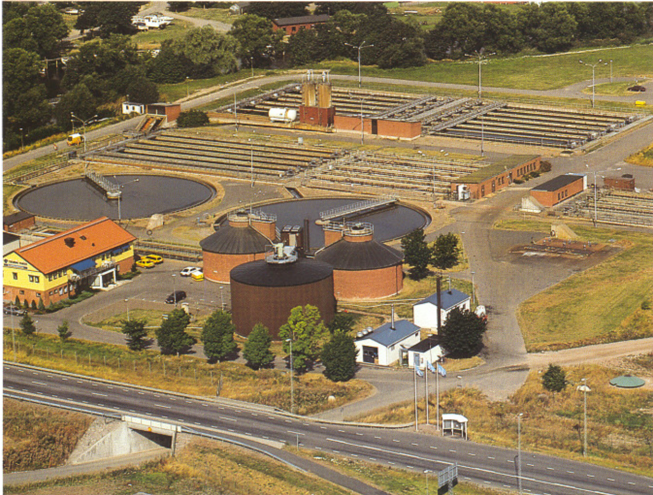
The plant at Nykvarn is one of the three water supply and sewage plants at Tekniska Verken which has a new monitoring system supplied by Cactus Automation. The Nykvarn plant succeeded in reducing nitrogen in built-up wetlands at an early stage. Some 200,000 residents of Östergötland region have their water treated at Nykvarn.
